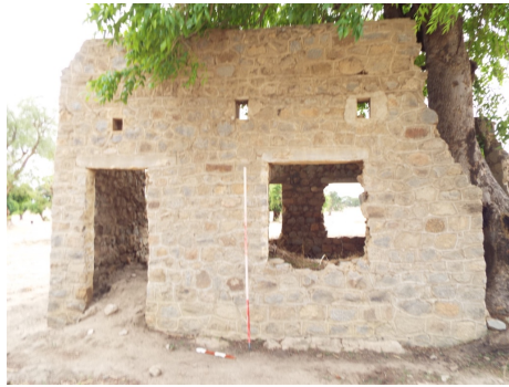
Plate 1: Dilapidated Court building
