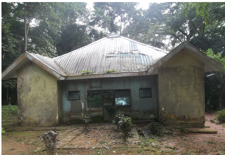
Plate 1: Showing dilapidated accommodation facility in Okomu National Park. Source: Field Survey, 2018
